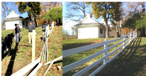
Eagle Scout candidate John Riley from troop Paoli 1 made a major contribution to the appearance of the Gatehouse and Lorimer Preserve. John's project was to restore the badly dilapidated 100-yard fence that borders the driveway leading to the Gatehouse and farm.
